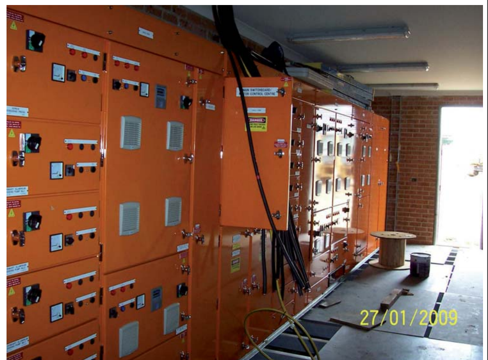
Electrical Switch Room - main witchboard installed
