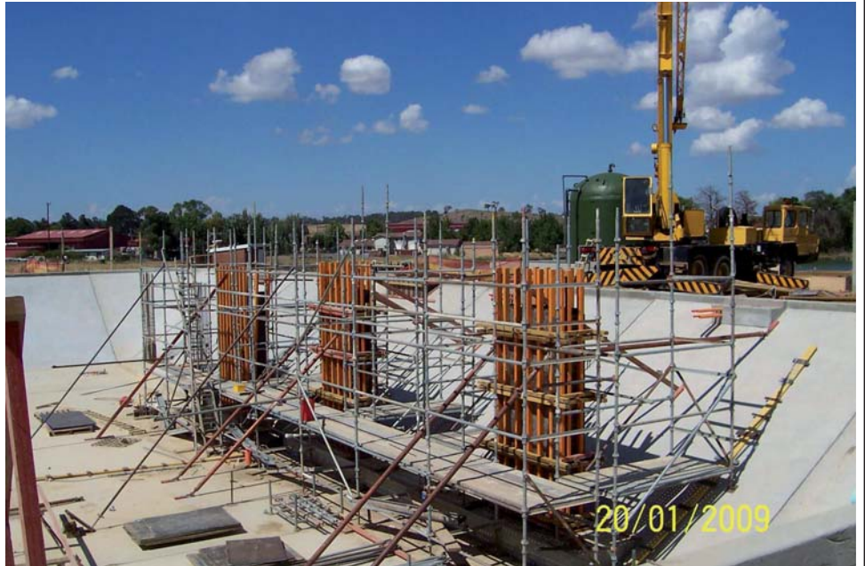
IDEAT - formwork for concrete columns for decant trough and aerator walkway supports
